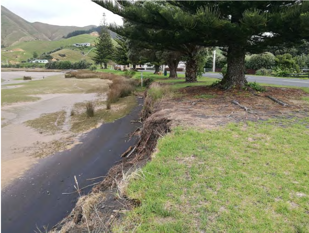
Figure 37: Bank erosion fronting the Esplanade. The erosion occurs primarily where the bank does not have a high tide dry beach to seaward. Locals advise that the erosion was primarily caused by waves.
